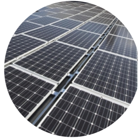
Desire to Increase Onsite Renewable Energy
